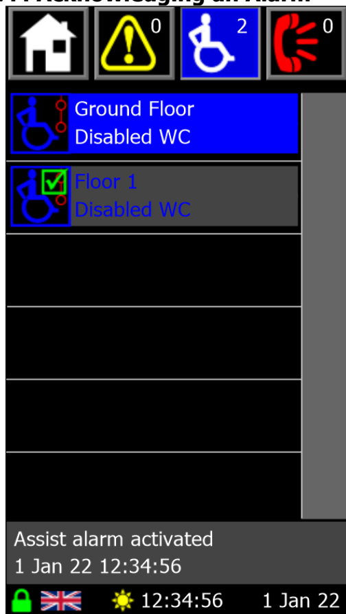
Figure 19 - TMS3 Alarm Screen
